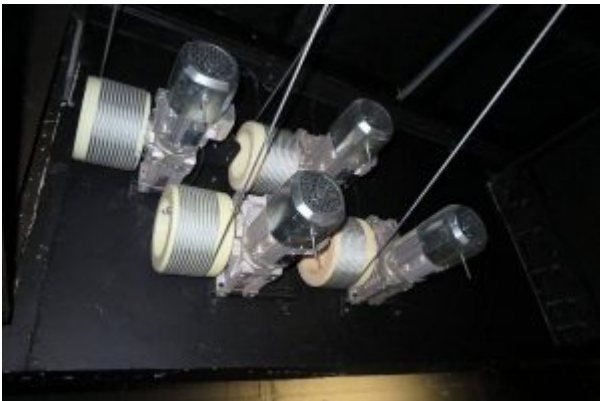
Motorised winch units
